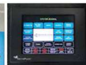
Touch Screen Multiplex System
