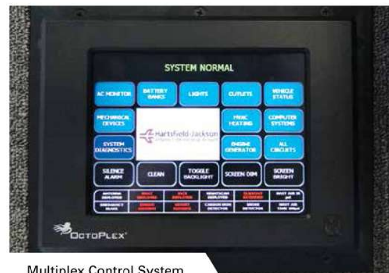
Multiplex Control System
