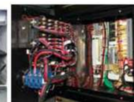
Custom Designed and Built Power Panels and Wiring Harnesses
